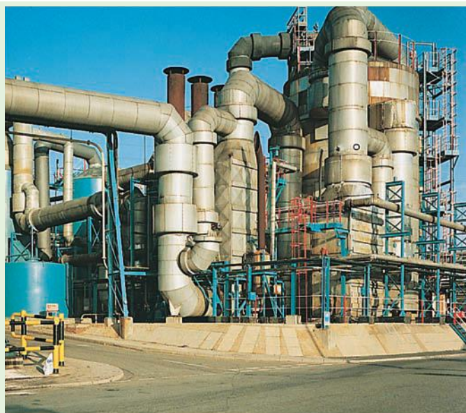
Figure 12.7 A Contact process plant used for making sulfuric acid.
