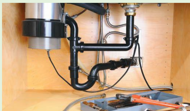
Figure 14.17 These pipes are made from PVC.
