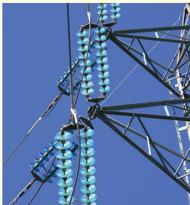
Figure 3.39 Ceramic discs prevent short-circuits in the national grid.
