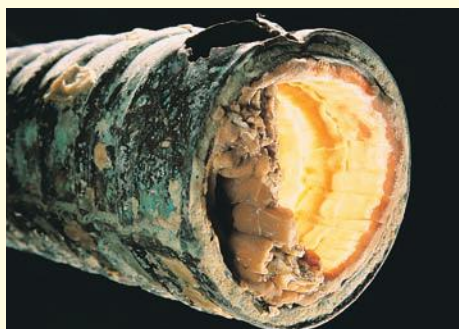
b The thick deposits of limescale can be seen in this hot water pipe. Figure 11.33
